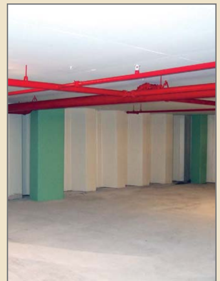
Finished parking garage with exposed sheet pile as the permanent wall element
