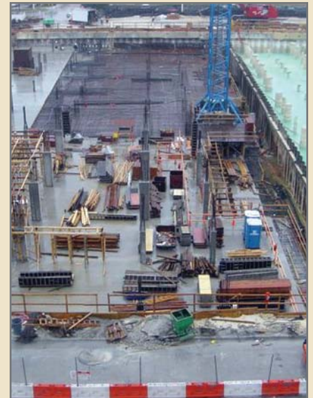
Excavation site: temporary sheet piles were used to partition sections for different construction phases
