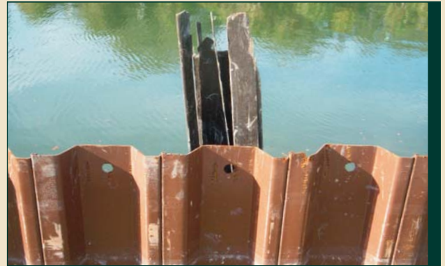
Steel sheet pile replacing failed FRP at installation
