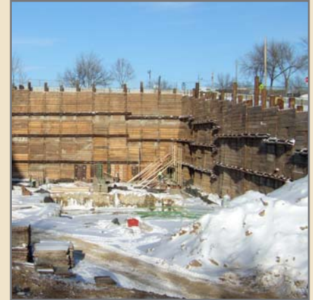
Typical beam and lagging shoring application constructed with materials from Skyline Steel
