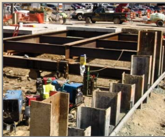
Vertical and cross bracing beams supplied by Skyline Steel for support of excavation
