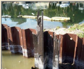
XPS replacing failed composite sheet pile
